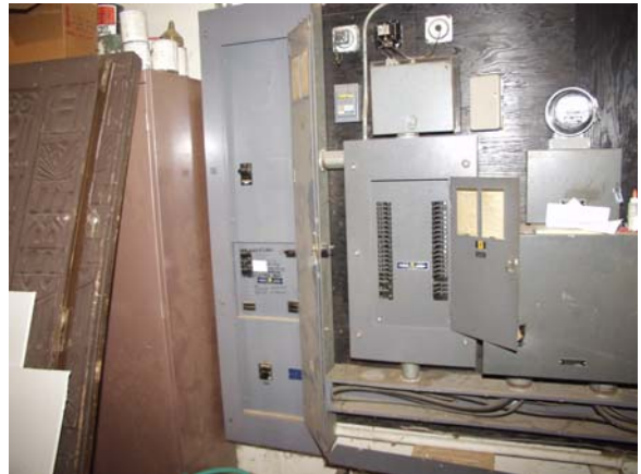
Main distribution panelboard at left, serving three subpanels, one of which is at right..
