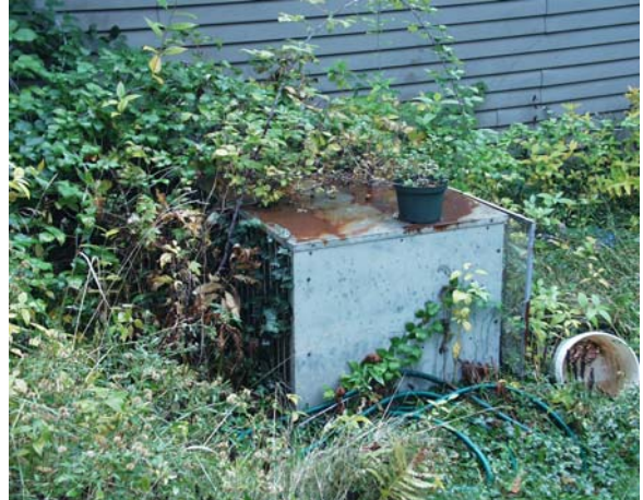
Section 3 air conditioning condensing unit (not operational).
