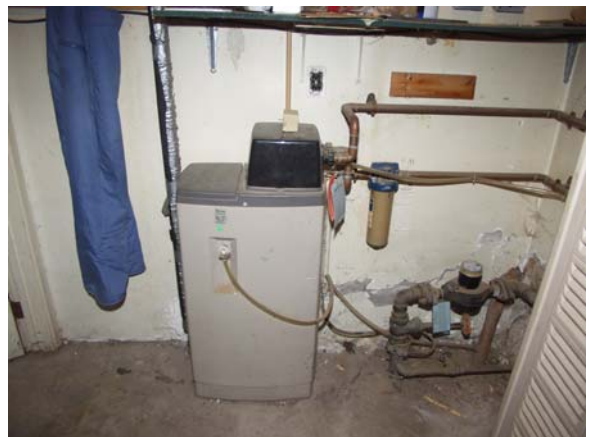
Water softener. Existing domestic water meter is to the right near the floor.
