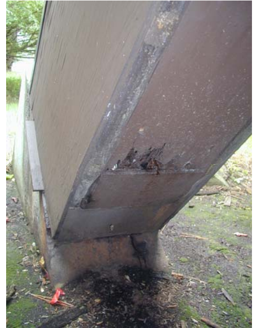
Decay at valley rafter bases and structural reinforcement.
