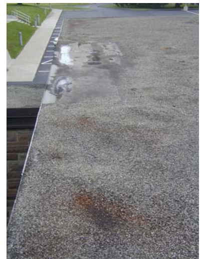
Ponding at roof edges.
