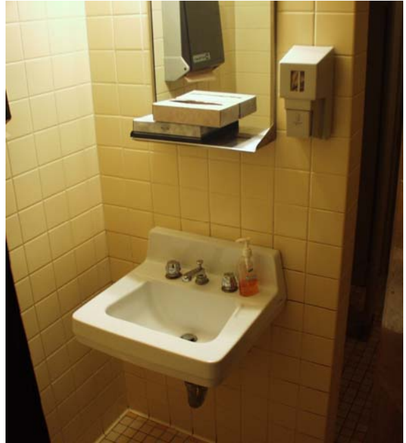
Section 3 bathroom. ADA compliance is not really practical in this small space.
