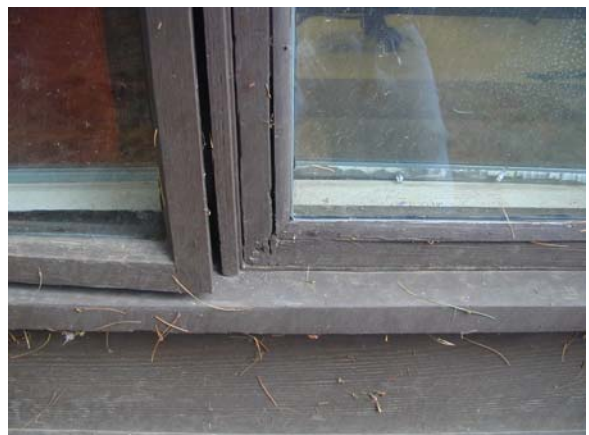
Sash detail of west facadecasement showing aging and repair.
