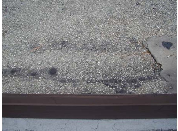
Blistering and patching near roof edges.
